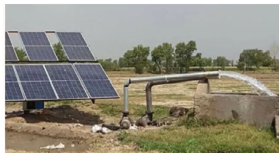
Fig. 4. Solar PV driven tubewell.
