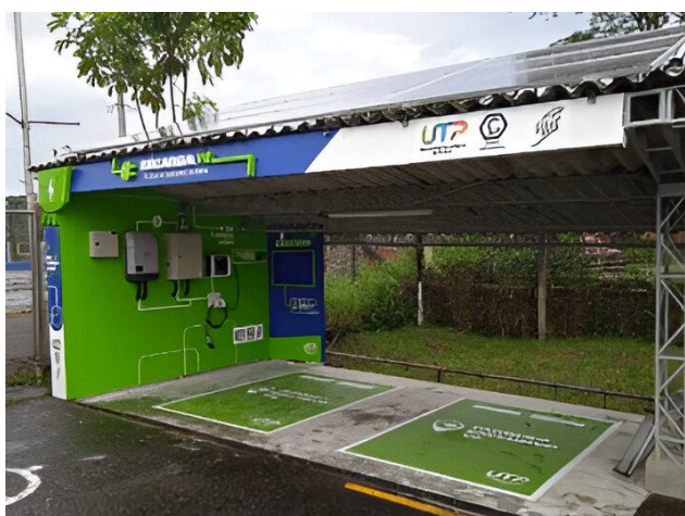
Fig. 5. Final Presentation of PV electric charging station
