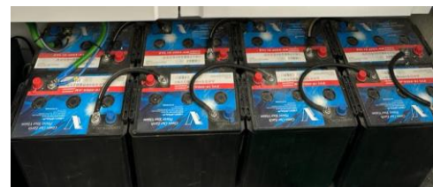
Fig.5. Batteries installed at GEDERlab.
